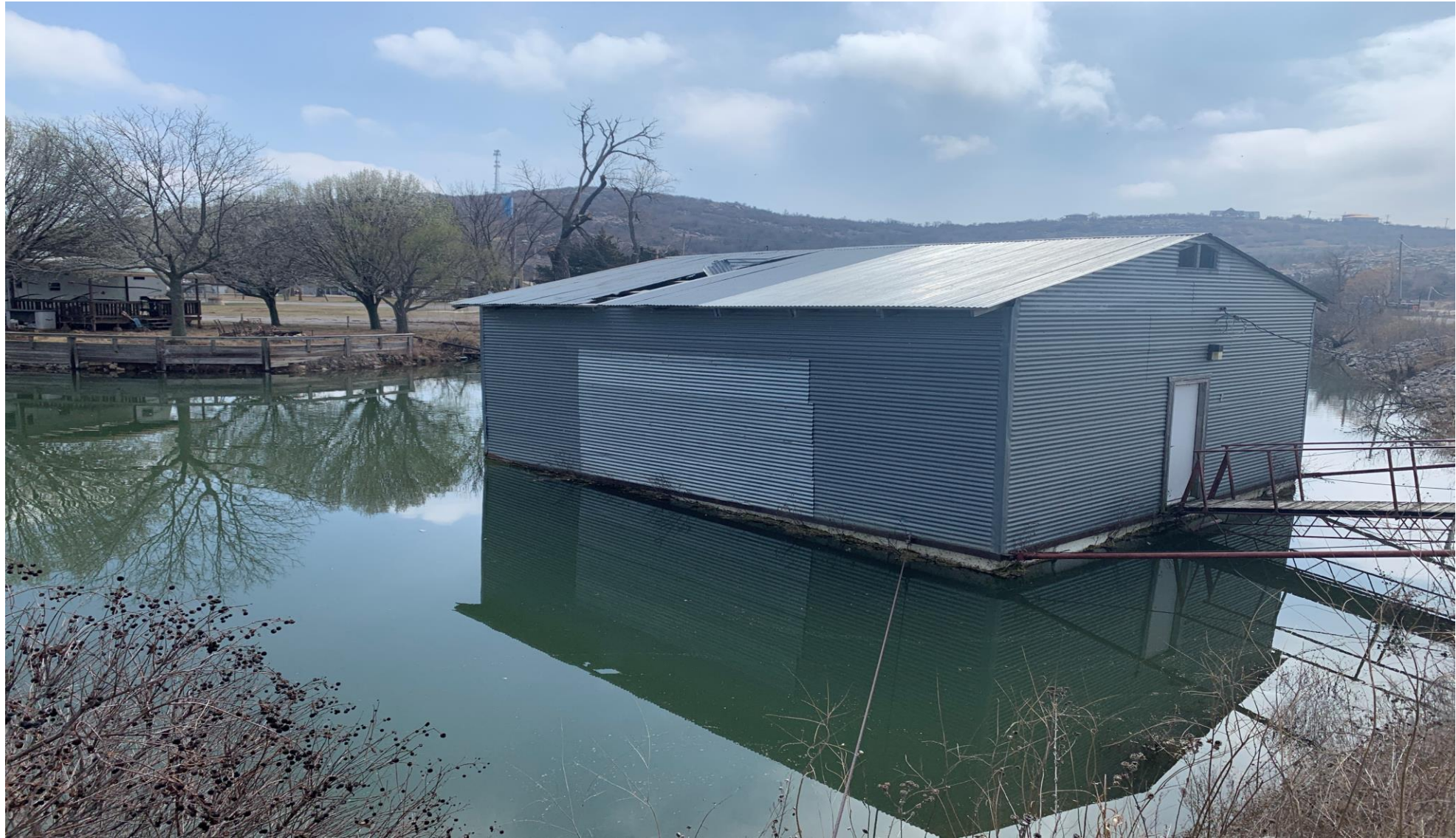
Wet Slip Photo 2
